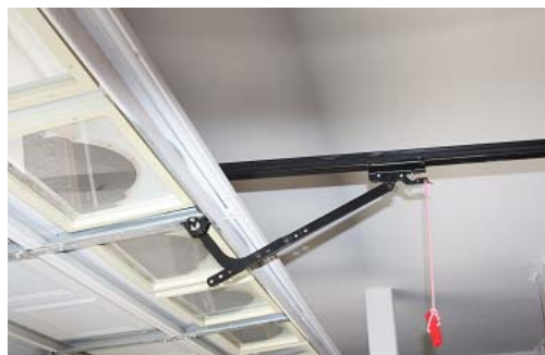
The garage door is lifted into the open position.
