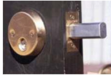
Cylinder too wide
